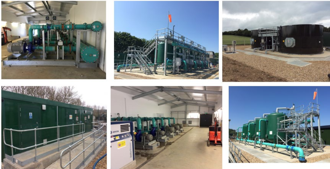
Image 1. Clockwise from L-R, Main building internals showing High-lift pumps, Backwash pumps, Air Scour blowers, Pressure filters, Dirty Washwater Tanks, Chlorination Kiosk, Main Building and Pressure Filters.
